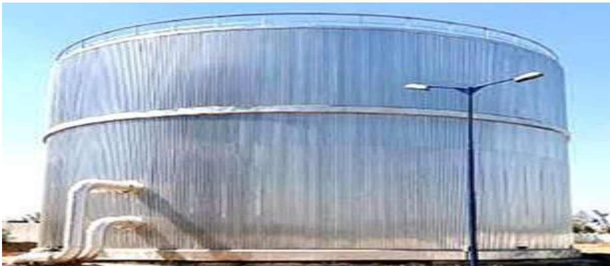
“Figure 8. TES tank at DCP-1 [2]”.
