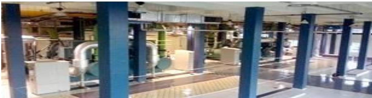
“Figure 7. 10,000 TR chillers at DCP-1 [2].”
