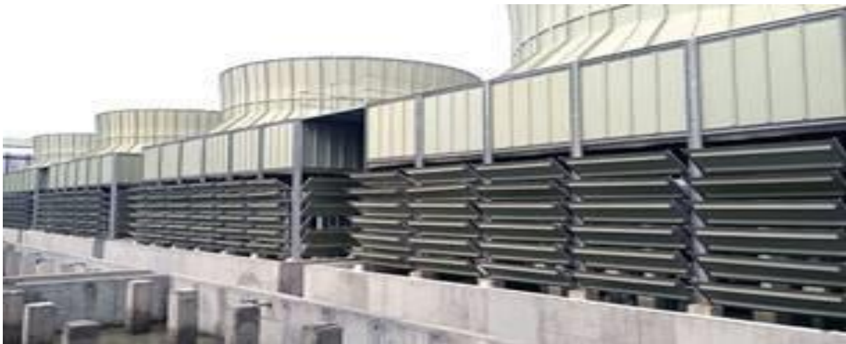
“Figure 10. Cooling towers [2].”
