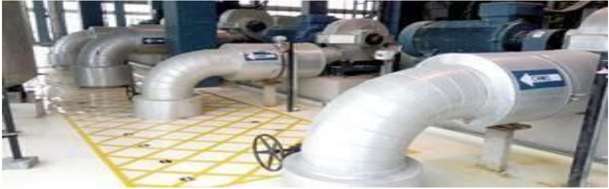
“Figure 9. Chilled water pipe routed below the ground trench [2]”.
