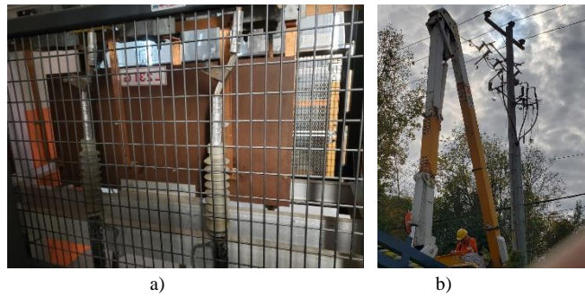
Fig. 11 Substation feeder cell a) and cable aerial outlet b) were UD 1 and UD 2 have been installed
