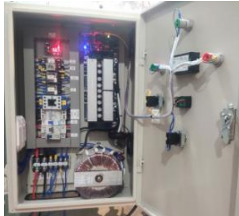
Figure 3. Hybrid generator control box
