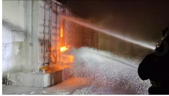
Fig. 3. Photograph of the Scene of the Fire Accident at the Energy Storage Station in Taichung, Taiwan.
