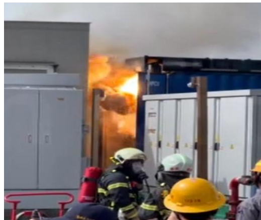
Fig. 4. Photograph of the Fire Scene at the Energy Storage Cabinet in Orchid Island Power Plant.
