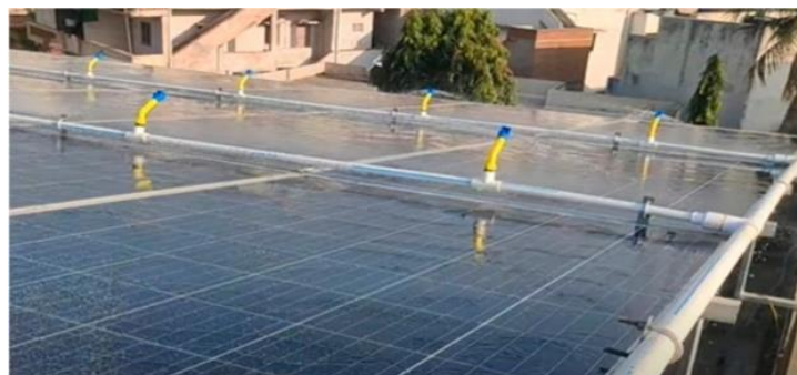
Fig.3 Cleaning systems of various photovoltaic arrays equipped with nozzles.
