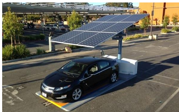
Figure 1. Solar Power EV charging Station
