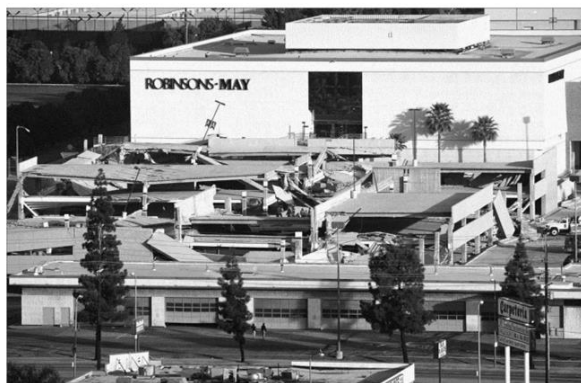
Figure 2. Diaphragm failure in the parking structure at the Northridge Fashion Centre during the January 1994 earthquake in Northridge, California (James, 2019)
