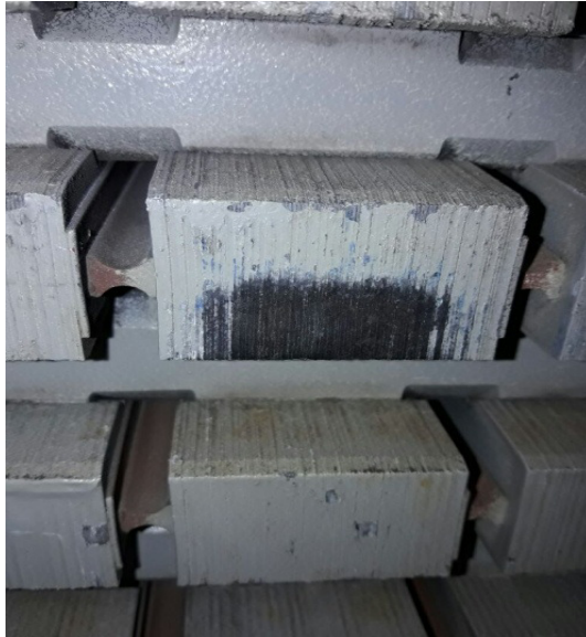
Fig. 4. Molten lump of stator winding coming in contact with slot-tooth, leaving a mark.
