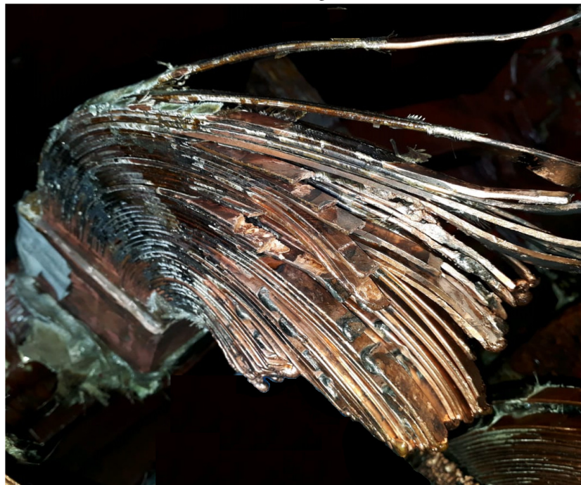
Fig. 6. A damaged coil showing burnt strip conductors in a typical high voltage alternator (Courtesy: Proclaim).
