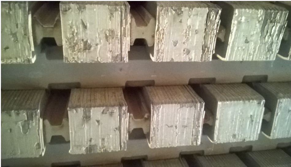
Fig. 2. Start of Loosening of Core stampings in 150 MW alternator.
