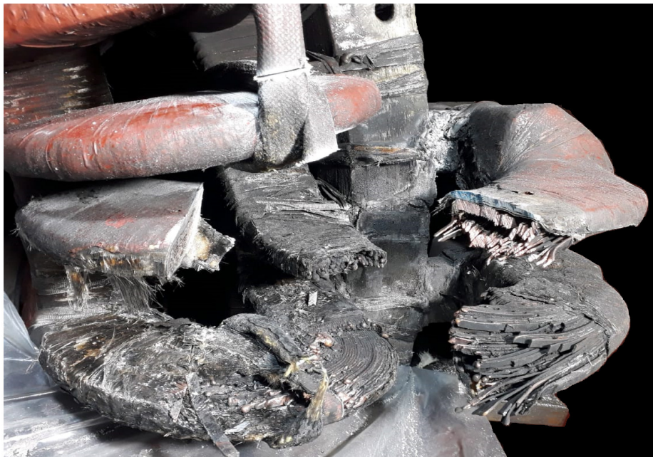
Fig. 9. Nose Joint Failure.
