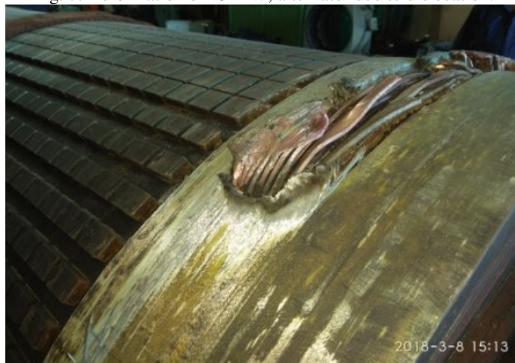
Fig. 8. Puncturing of glass insulation covering the overhang portion of the rotor due to dislocation of stator winding causing direct contact with the rotor.
