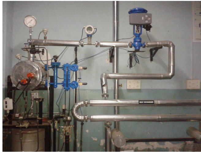
Fig 7. Boiler Heat Exchanger Setup
