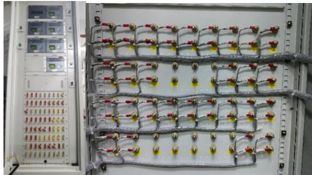
Figure 1: Physical Image of Cabinet
