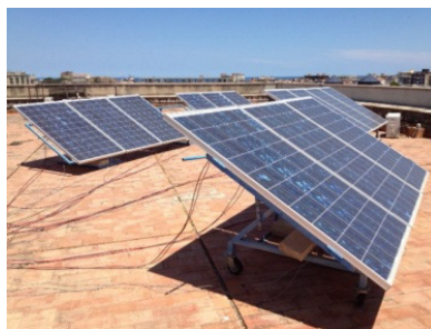
Fig. 6 Experimental setup with 12 panels individually connected to the reconfigurator.
